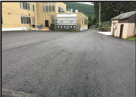
The Chenango Bridge west parking lot asphalt has been removed and new asphalt binder is down. The asphalt top has since been installed and the parking lot is complete.
