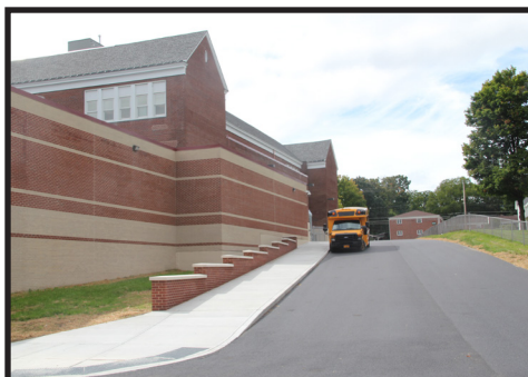
A new concrete walk along the PDE bus loop is complete. Asphalt at the bus loop was removed and new asphalt binder was installed. The asphalt top has been installed and the bus loop is complete.
