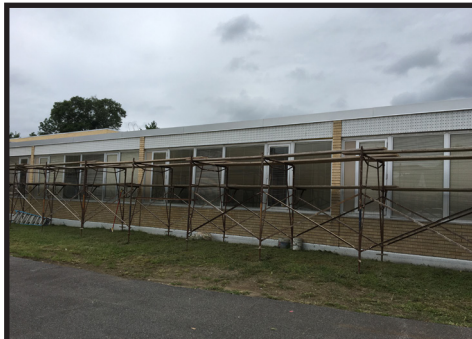
At Chenango Bridge, porcelain panels above the windows at the rear of the building have been removed and a new thin brick system will be installed soon.
