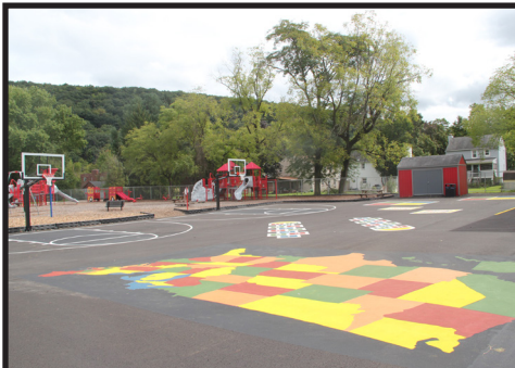
Asphalt at the Port Dickinson play area has been removed and new asphalt has been installed.
